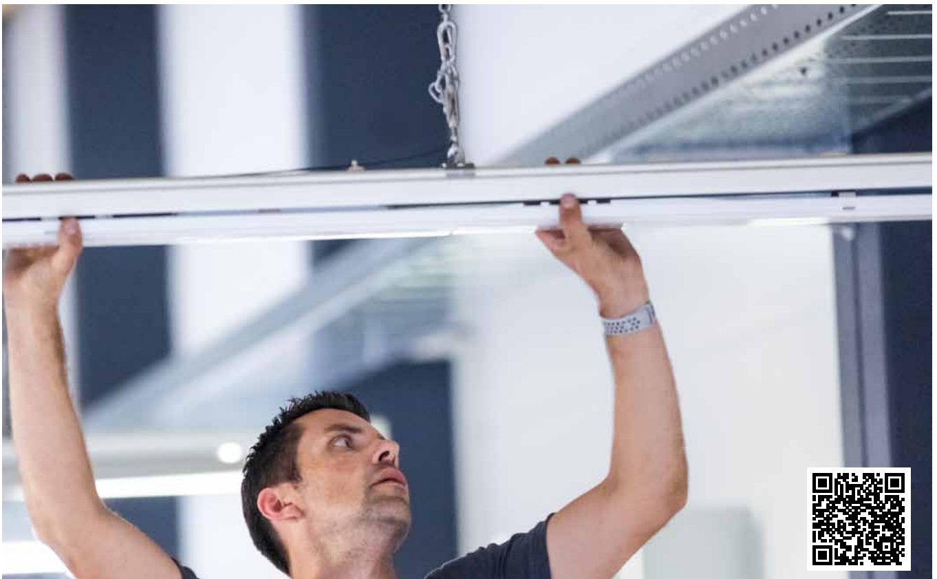
From old to new during running operation – experience the lighting refurbishment at Wache Lübeck GmbH
