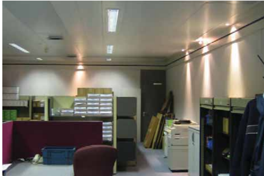
Figure 2.2 shows some decorative spotlights mounted too close to a perimeter wall due to poor coordination with the ceiling arrangement.
