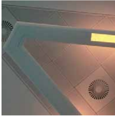
Figure 7.1 Supply diffuser and suspended luminaire
