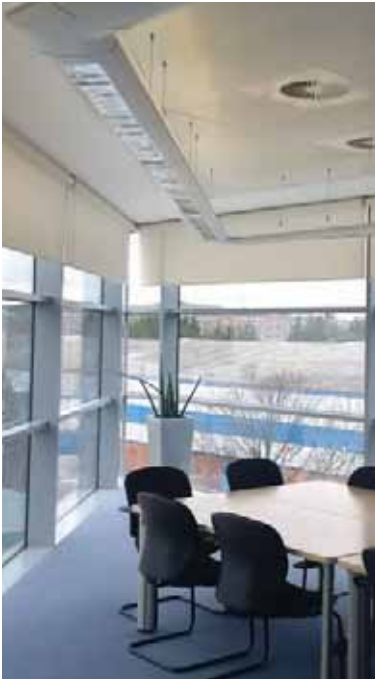
Figure 6.15 Combined direct and indirect lighting installation
